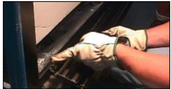
Figure 24 - Control Access Panel
